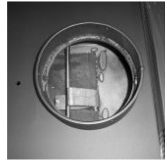
VIEW OF BYPASS DOOR AND CRANK THROUGH COLLAR
