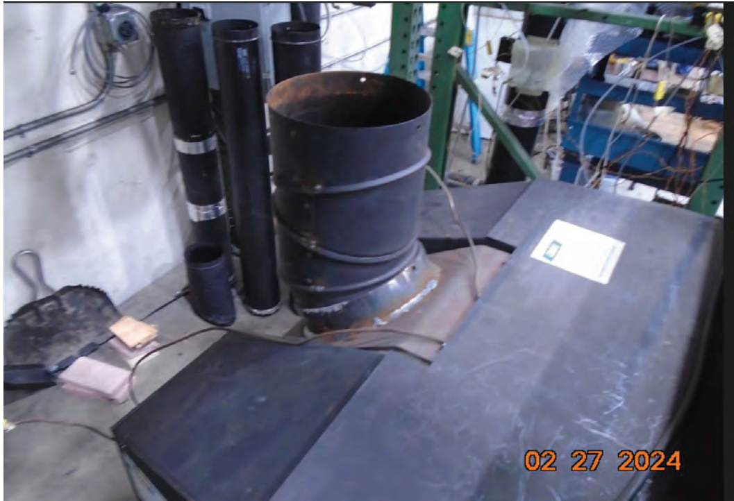
Figure 9 - A 30° elbow was required by this appliance
